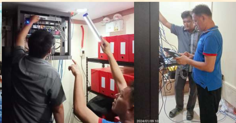
Regional Office — Repair of internet connectivity and configuration of voice over internet protocol phone (VoIP) at the Server Room
