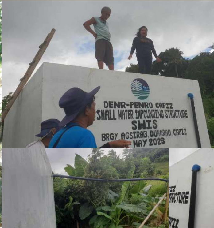
PENRO Capiz—Completed SWIS in Brgy. Agsirab, Dumarao, Capiz during the monitoring on November 28-December 01, 2023
