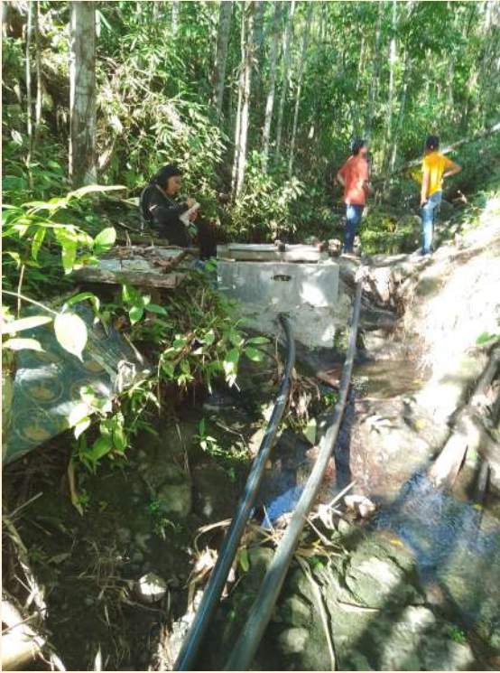
PENRO Capiz—Constructed spring box connecting to the SWIS in Brgy. San Antonio, Tapaz, Capiz during the monitoring on November 28-December 01, 2023
