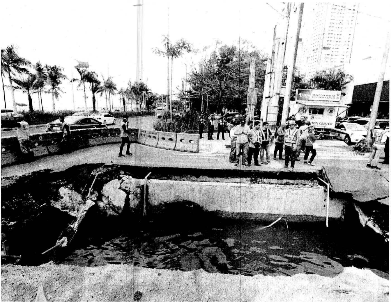
HOW BIG IS THE HOLE. – The size of the big hole that formed after a 14-wheeler truck carrying sand sank in this portion of the street at the intersection of Remedios Street and Roxas Boulevard in Manila Sunday is being measured through Real Time Kinematics (RTK) by Department of Public Works and Highways (DPWH) Engineer Jojo Barrios. (All Vicoy)
