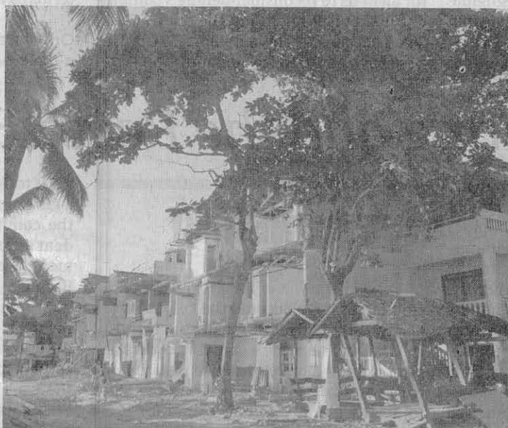
DEMOLISHED Sections of a beachfront hotel in Boracay are demolished over violation of easement rules as the government continues the environmental rehabilitation of the resort island in Malay, Aklan province. —ROBERT JAWORSKI L. ABAÑO
